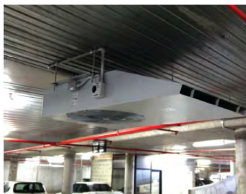
Example of a Jetvent Fan Installed in a car park.
